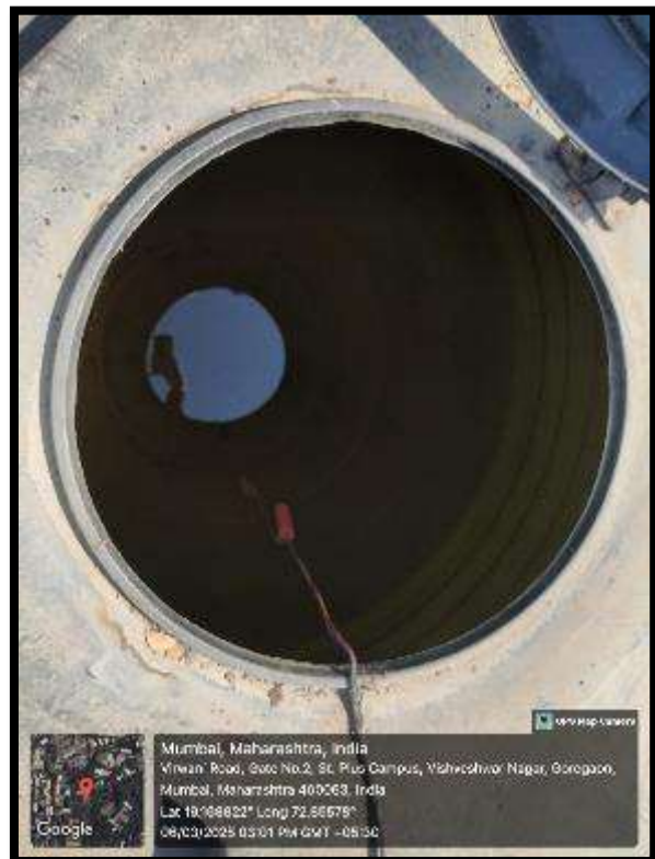
Water level indicator installed in water tank
