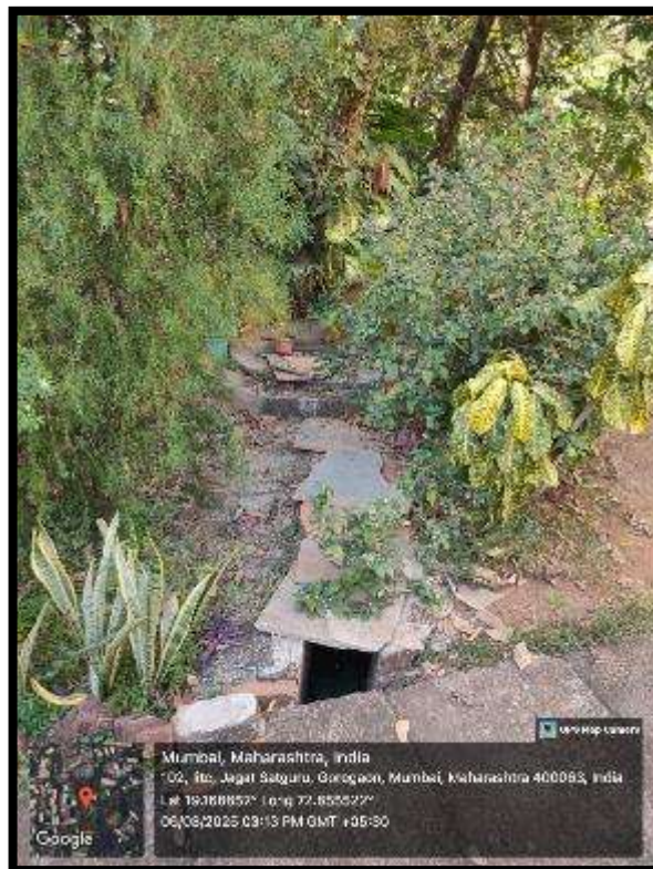
Rain Water Harvesting in Extension Centre
