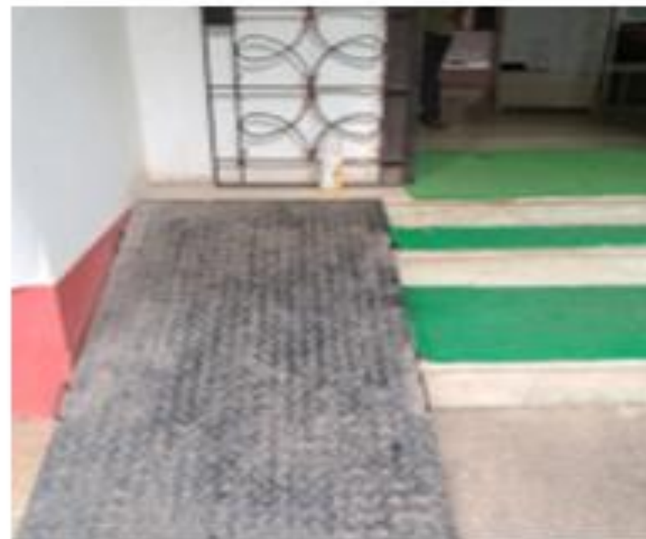
Ramp for Wheel chair access
