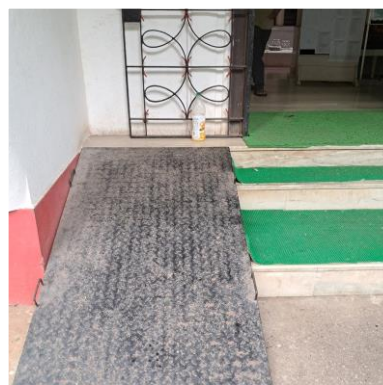
Ramp for Wheel chair access
