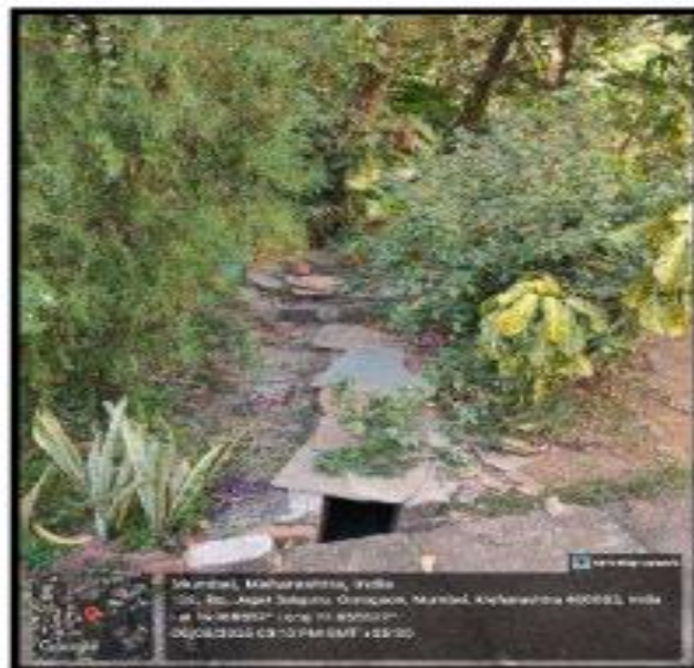
Rain Water Harvesting in Extension Centre
