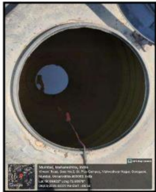
Water level indicator installed in water tank
